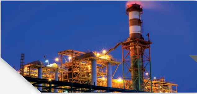
Gaz ve Petrol Gas and Petroleum
